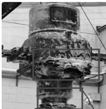
图1 试品试验后的局部破损照片 Fig. 1 Picture of partial damaged test sample after test
